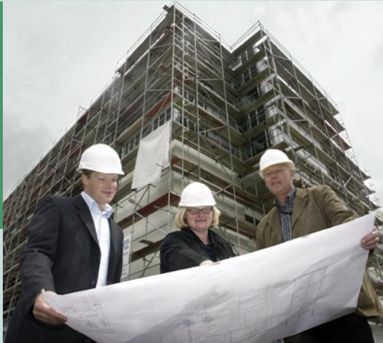
Construction Site Supervisor, Harald Broessel (left) with Sub-project Managers Esther Seidel and Peter Fieber outside the new filling and lyophilisation facility being built in Marburg. Coagulation therapies used in the treatment of bleeding disorders such as haemophilia and von Willebrand disease will be manufactured in this new complex.
