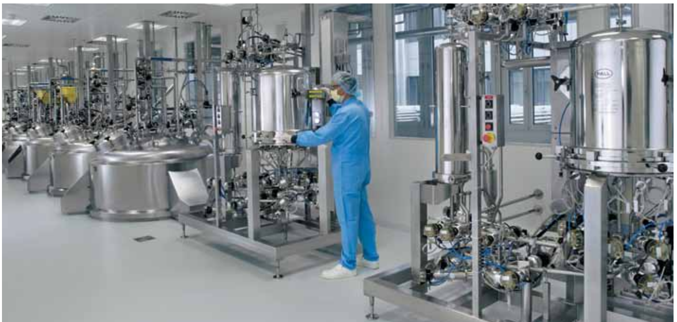
Inside the IgLAB bulk manufacturing facility in Bern where chromatography and virus filtration operations are carried out for Privigen® and Hizentra®.
